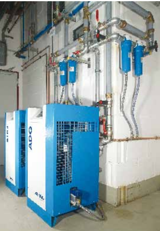
Each compressor has its own preparation line
