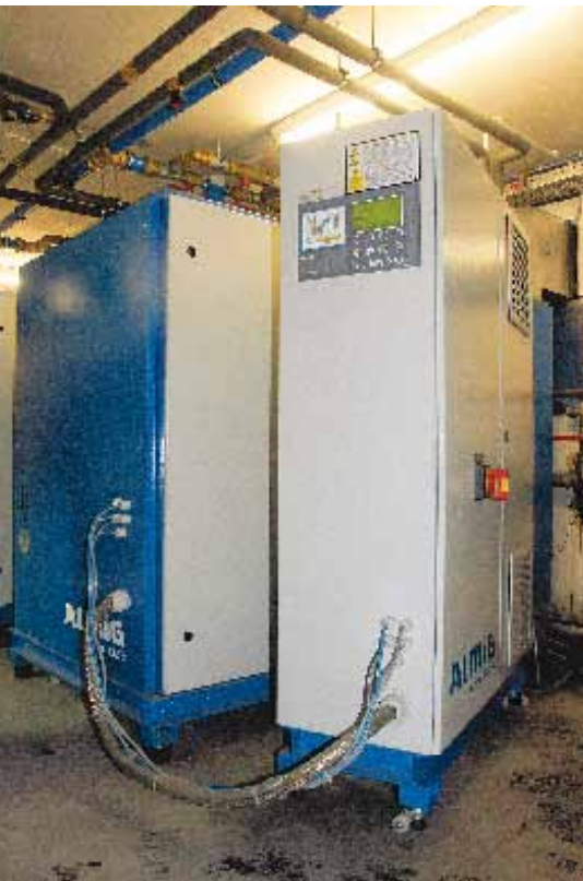
The limited space required the control cabinets to be separated from the compressors and positioned on base frames that could be moved on castors
